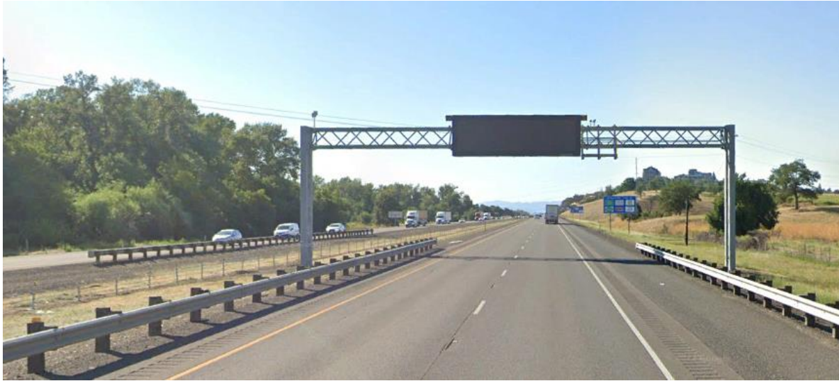
Figure 9. VMS on I-5
